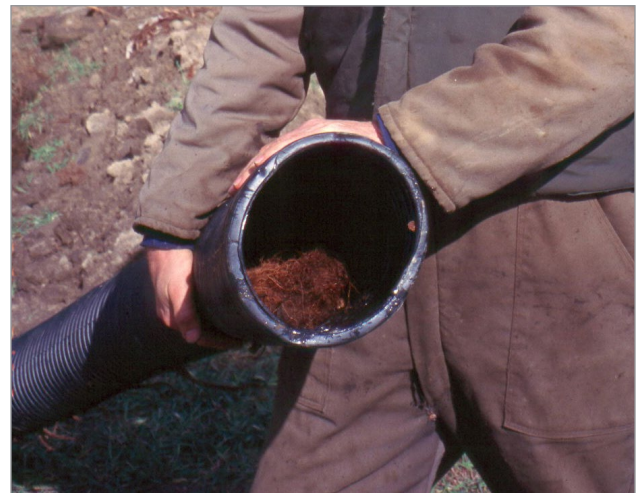
Figure 4. A large section of drain pipe is plugged by roots from a large willow tree growing 30 m away. The plugged section must be dug up and replaced with a new section of pipe. (Photo credit: Long Point Conservation Authority, Ontario)
