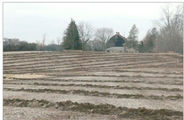
Figure 3. Parallel rows of back-filled soil show where drain pipe was recently installed in this field.
