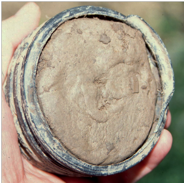
Figure 1. At first glance, this drain pipe appears to be plugged by soil.
