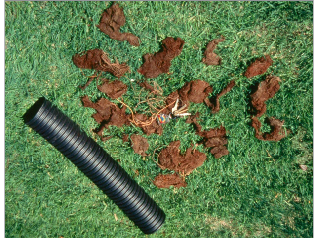
Figure 5. Masses of root pulled from the plugged drain are from nearby peach trees. While it is rare, roots of dry-site trees, such as peach, can also plug pipes, as shown here.
