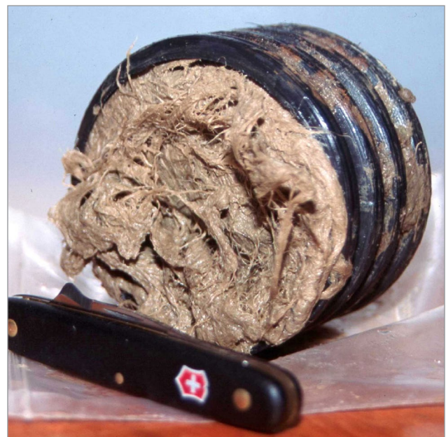
Figure 2. Rinsing soil away from the section of pipe shown in Figure 1 shows it is also plugged with dense fibrous roots, holding small soil particles flowing in the drainage water.
