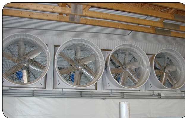
Figure 6. Fans provide power to move and exchange air.
