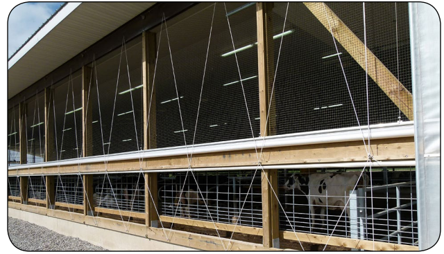
Figure 3. Sidewall inlet with bird screen on the top section.
