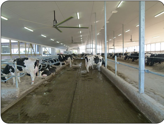
Figure 8. Place HVLS fans over the free stalls for cooling.
