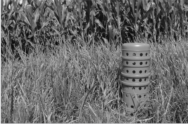
Figure 4. A catch basin used to drain surface water.
