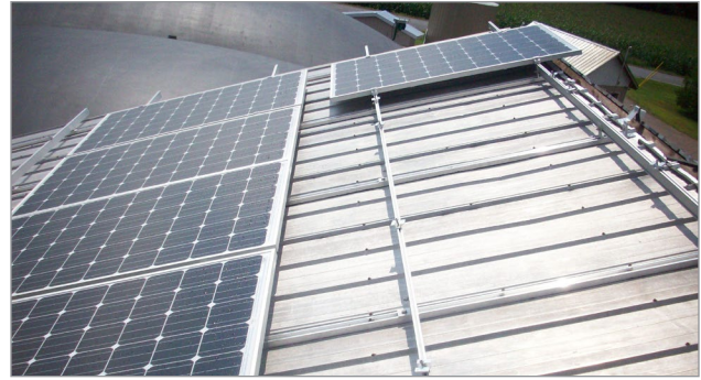
Figure 3. A solar panel installation of crystalline silicon modules with rows for maintenance access and ventilation.
