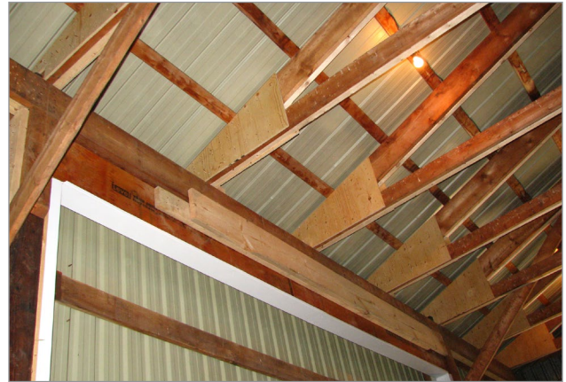
Figure 10. Plywood reinforcing provides additional support in this storage shed.
