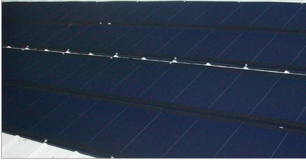
Figure 12. A thin film installation where the material has been directly applied to the roof.
