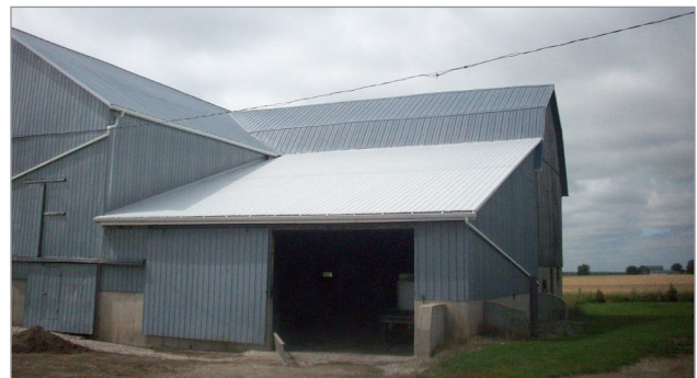
Figure 5. A rooftop with a complex loading pattern due to the different parts of the building coming together and the use of eave troughs.
