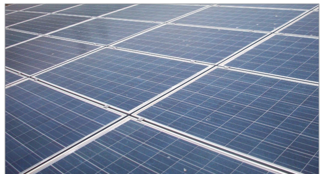
Figure 4. A solar panel installation where the crystalline silicon modules are installed tightly together, approximately 19-mm gap in between rows.
