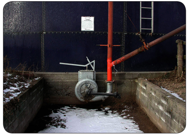
Figure 3. A side-mounted liquid manure pump on an above-ground, steel manure storage.
