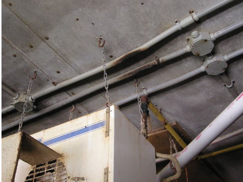
Figure 3.14. A box heater properly suspended on four jack chains. Note that a faulty gas valve resulted in charring of the electrical conduit. (Photo credit: R. Drysdale, Farm Mutual Reinsurance Plan)
