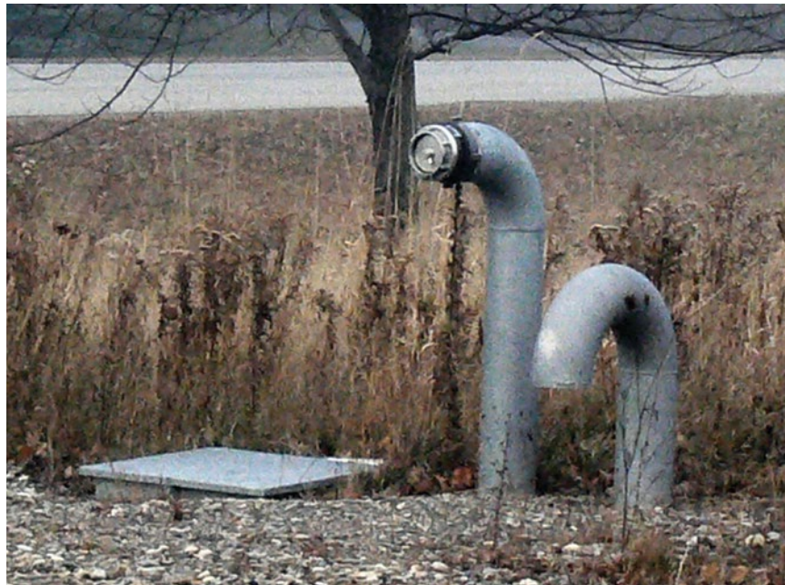
Figure 4.5. Dry hydrant showing all features.
