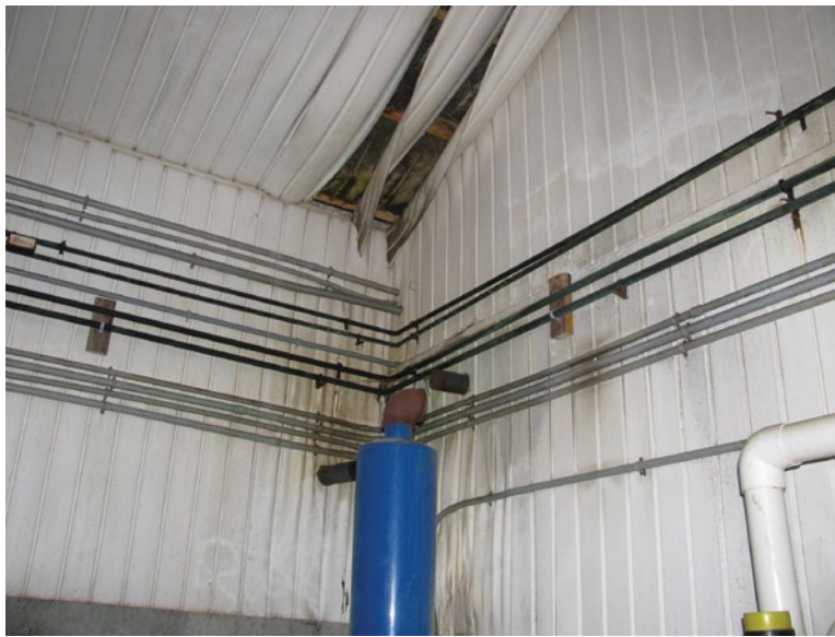
Figure 3.11. Melted vinyl sheathing on ceiling. Note the lack of backing behind the vinyl leaving the attic space exposed.
