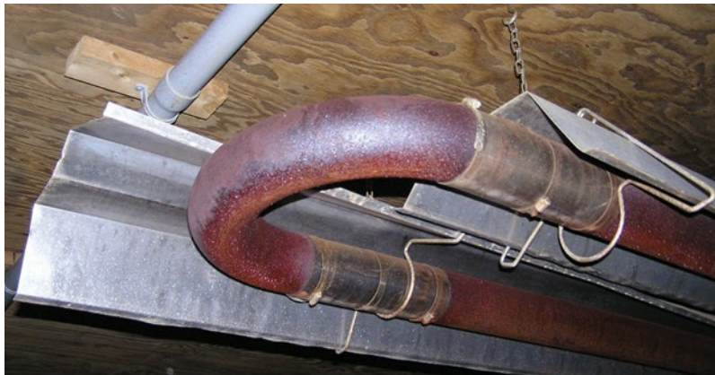
Figure 2.9. Radiant tube heater lacking heat shield. Note close proximity to combustibles (wood ceiling and conduit).
