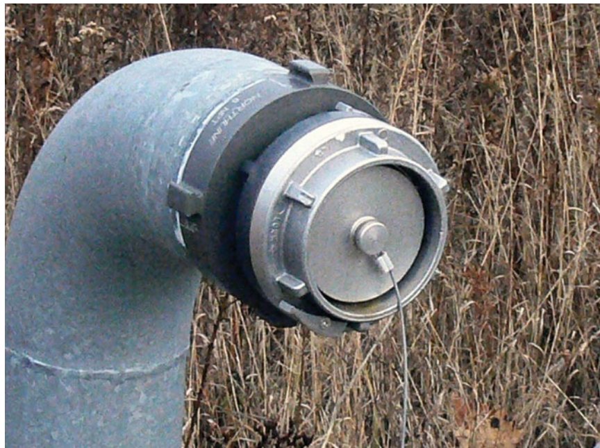
Figure 4.6. Dry hydrant standpipe connection.
