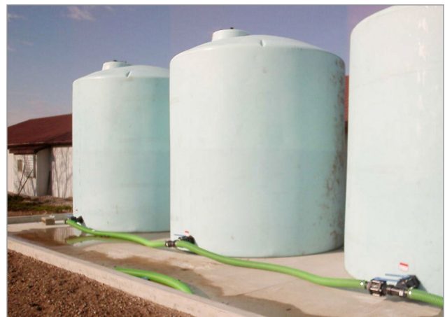
Figure 1. Poly tank farm with containment dike.
