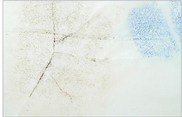
Figure 5. Tank showing evidence of crazing (in blue) and cracking (black) when coloured with a water-soluble marker.
