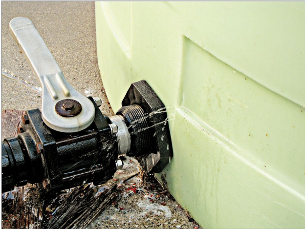
Figure 3. Stress cracking in poly tank beside the plumbing outlet, resulting in liquid loss.
