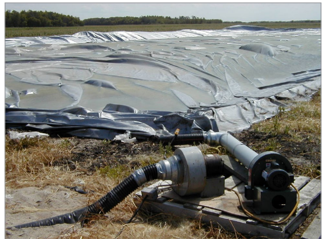
Figure 6. Negative pressure cover on an earthen manure storage.
