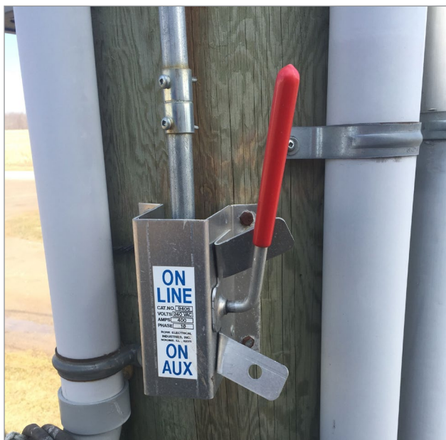
Figure 4. Example of a manual transfer switch mechanism for a portable generator, to disconnect utility power (“On Line”) from generator power (“On Aux”).
