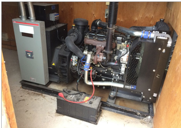
Figure 1. This self-contained engine-driven generator is permanently installed at a poultry farm and starts automatically when there is a power failure.
