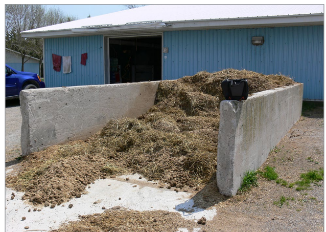
Figure 1. A 3-walled manure storage with reinforced concrete walls, located close to the barn.
