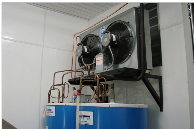
Figure 11. Heat reclaimer for pre-heating washwater.
