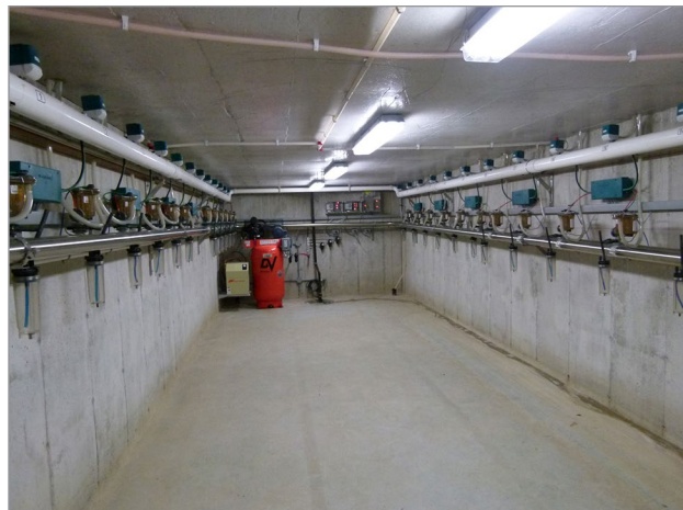
Figure 5. Installing pulsators in a basement in the milking centre will reduce parlour noise.
