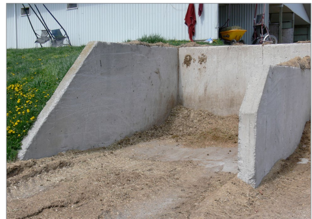
Figure 6. Storage in the side of a hill makes it easy to dump wheelbarrows. Install safety stops at the top edge.
