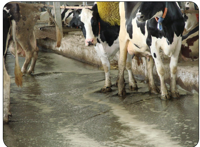
Figure 6. Flush system for cleaning cow alleys.
