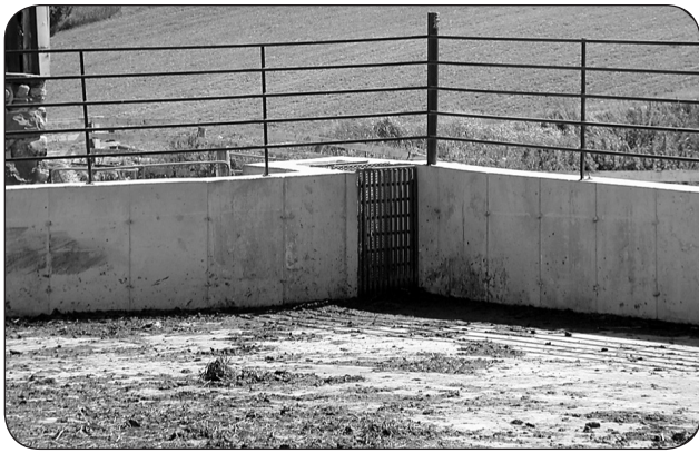
Figure 3. Placing three screens at the lowest point in the POCA limit the amount of solids reaching the holding tank and pump of the VFSS.
