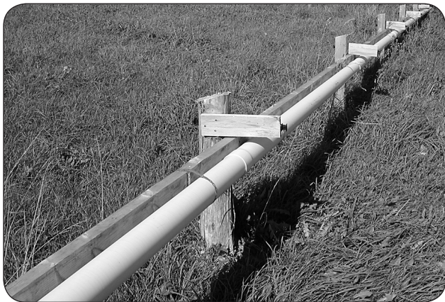
Figure 4. When the holding tank reaches a sufficient volume of runoff, the pump sends the liquid through a pipe that on this farm is 40 m (130 ft.) long with 1.9 cm (¾ in.) holes drilled every 4.5 m (15 ft.) to allow for an even distribution across the entire vegetated strip.
