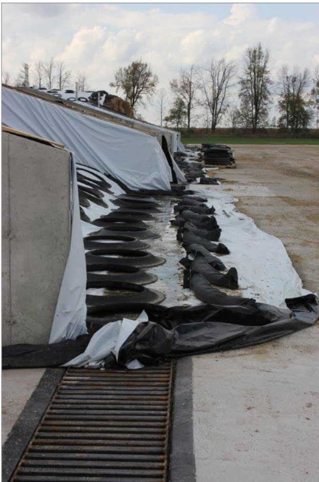
Figure 7. Collection trench in front of a filled bunker, only seepage can enter the trench.
