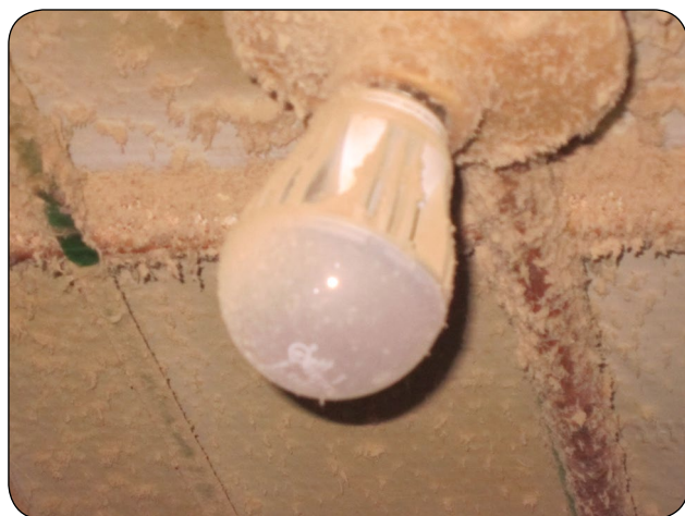
Figure 7. Edison-style LED bulb with heat dissipating fins covered in a layer of insulating dust. Source: National Poultry Technology Center, Auburn University, www.poultryhouse.com .
