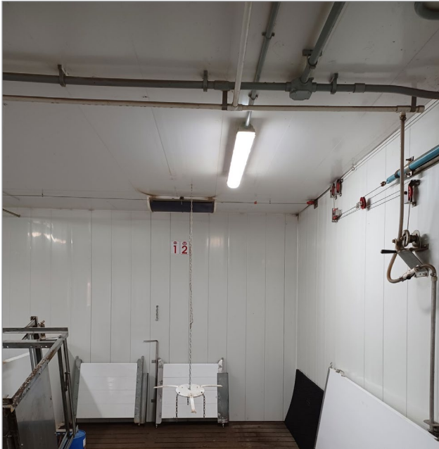
Figure 3. LED linear fixtures installed in a finisher barn.
