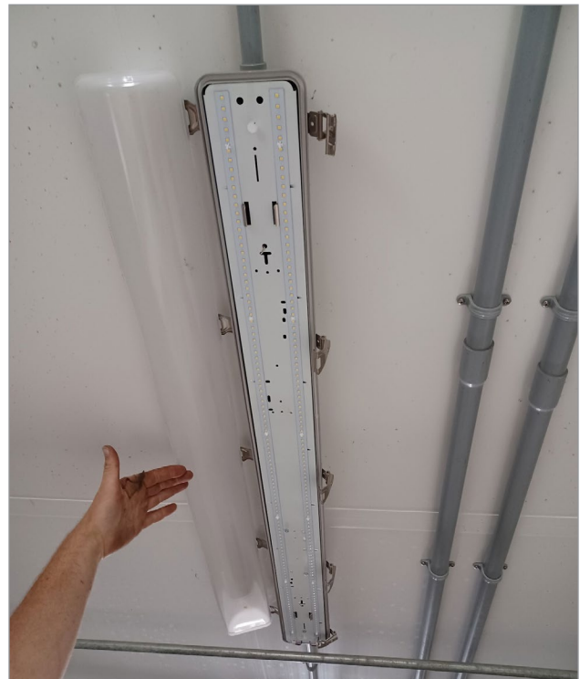
Figure 4. Inside an LED linear fixture. LEDs are solid state devices. Each square is a LED. Note the gasket for the lens, making this fixture vapour tight
