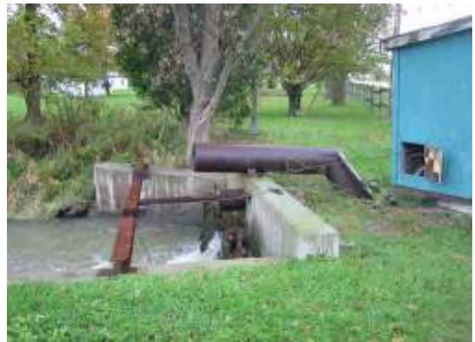
Figure A3-10. Station de pompage.
