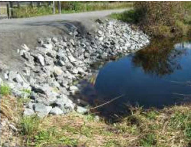
Figure B5-12. Hazeldean Road Drain – cross culvert under the Trans Canada trail.
