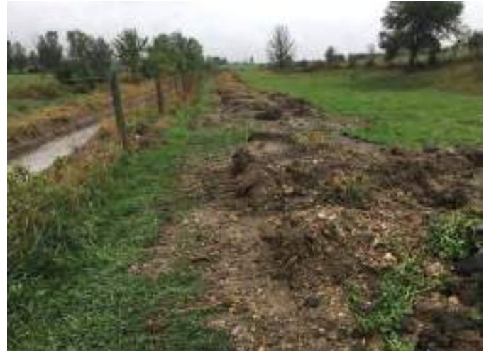
Figure A2-7. Excavated material spread to the right of the drain on farmland.
