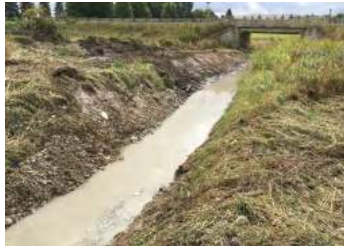
Figure A3-12. A bottom and left bank cleanout with vegetation remaining on the right bank.
