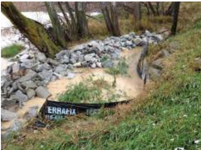
Figure B4-8. Turbid water in a drain due to erosion.
