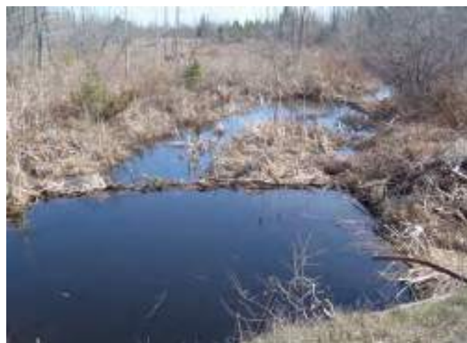
Figure B5-11. Hazeldean Road Drain – obstruction in the drain caused by beaver activity.
