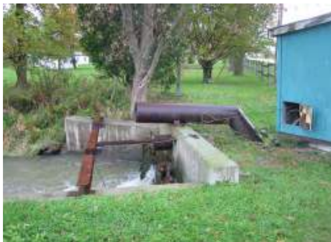
Figure A3-10. A pumping station. Source: Municipality of Chatham-Kent, Ontario
