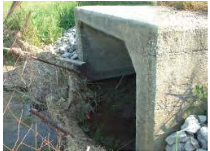
Figure A2-12. Farm fence obstructing the drain. Source: Bill Mayes, Norfolk County, Ontario
