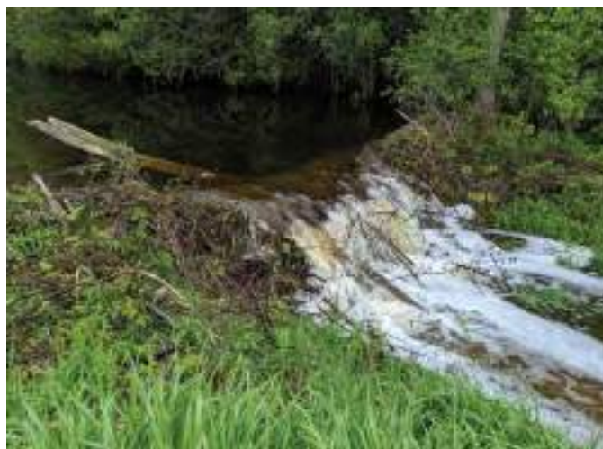
Figure A3-5. A beaver dam obstructing the flow of a drain. Source: City of Kawartha Lakes, Ontario
