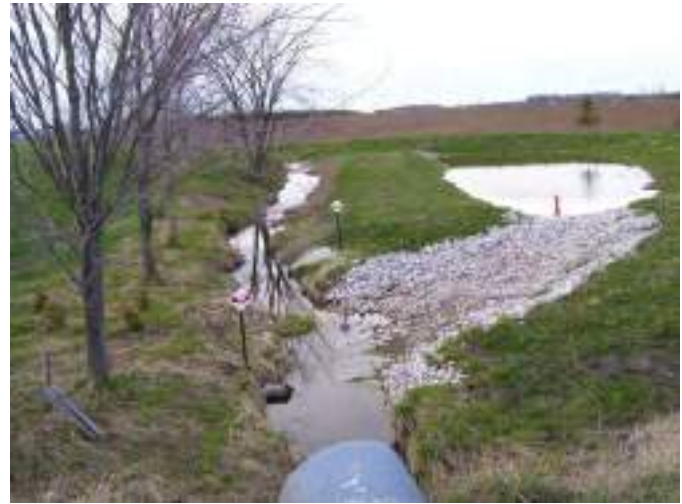
Figure B5-7. Steenstra Drain – Sediment trap after a high flow event. Source: Municipality of Central Huron, Ontario
