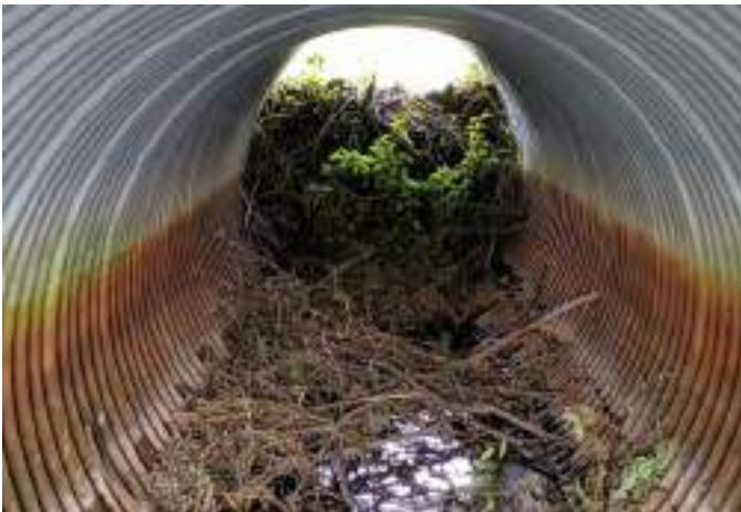
Figure A3-21. A beaver dam built on the upstream side of a culvert. Source: City of Kawartha Lakes, Ontario
