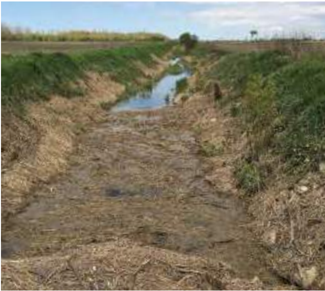
Figure A5-2. An obstruction in the drain to be removed by the property owner.
