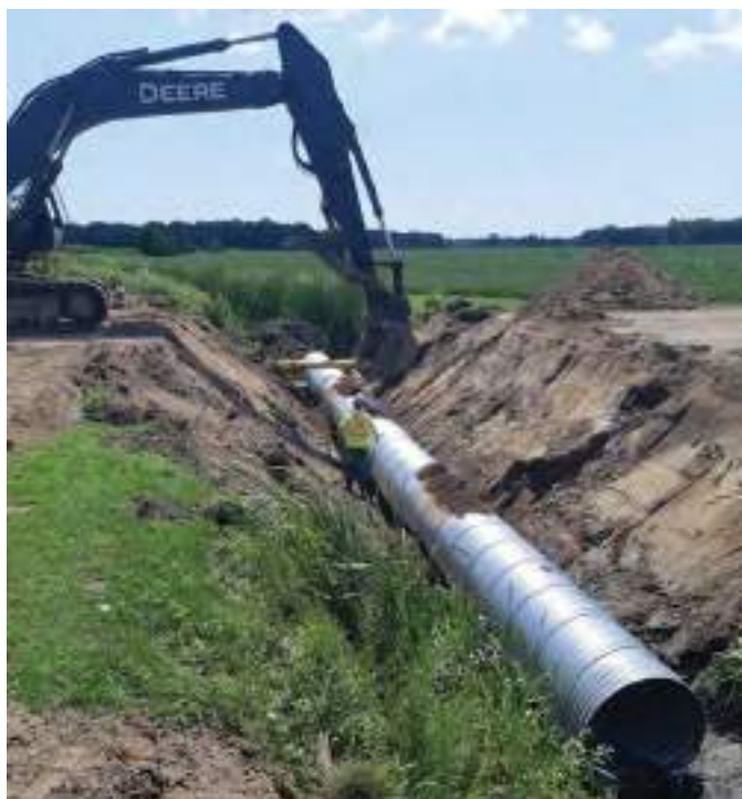
Figure A3-6. Placement of the new culvert as part of a crossing replacement.
