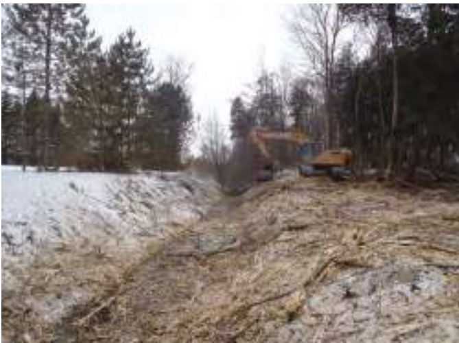
Figure A3-3. Brushing the drain bank. Source: Dietrich Engineering Ltd., Kitchener, Ontario.
