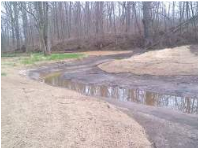
Figure B4-32. Rolled erosion control product installed on the banks of a drain.
