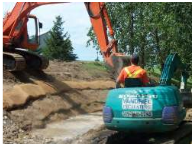
Figure B5-10. Steenstra Drain – Construction of the bioengineered channel bank. Source: Municipality of Central Huron, Ontario
