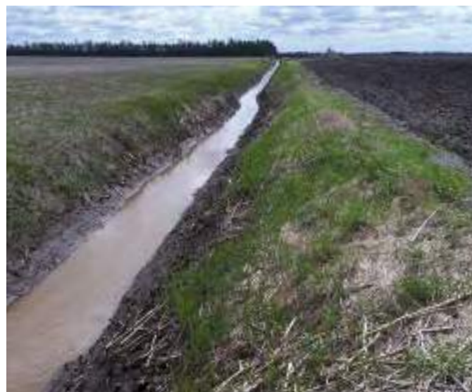
Figure A3-11. A bottom cleanout of a drain with vegetation remaining on the bank. Source: Leroux Consultant, Municipality of Alfred-Plantagenet, Ontario
