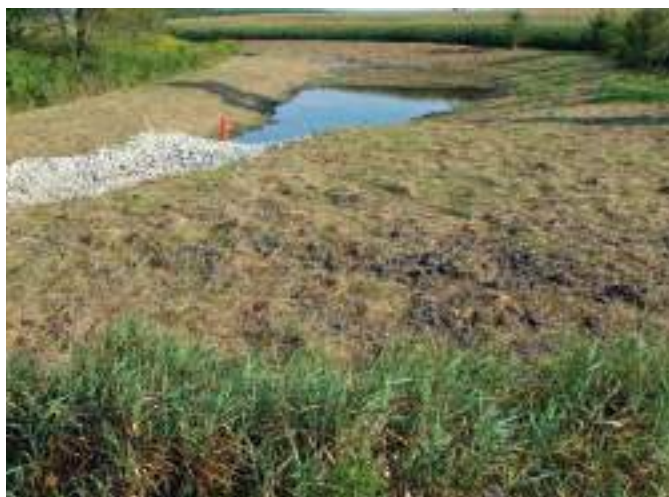
Figure B4-25. Straw/hay mulch spread on exposed soil surrounding a sediment trap. Source: Ausable Bayfield Conservation Authority, Ontario
