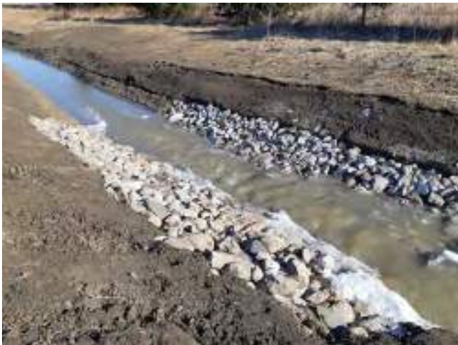
Figure B4-11. A water control structure (weir). Source: Municipality of West Elgin, Ontario
