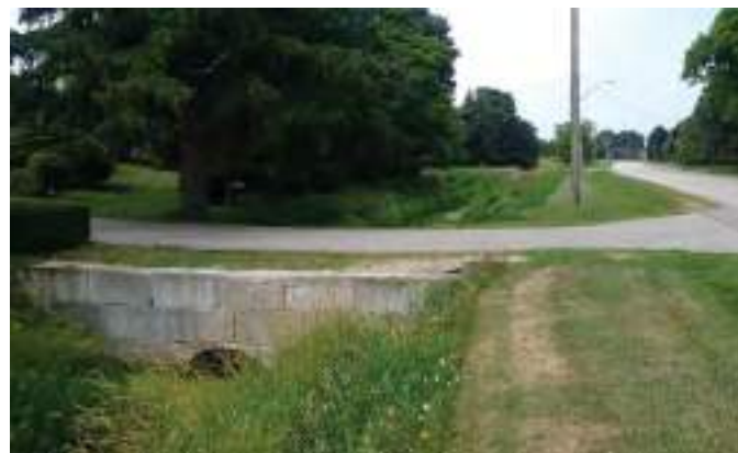
Figure A3-25. Access crossing over a drain. Source: Municipality of Chatham-Kent, Ontario
