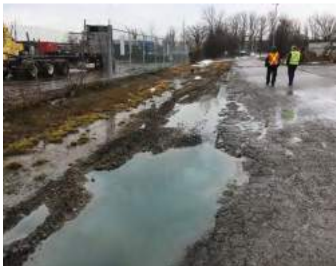
Figure B5-22. Southdown – drainage issue despite the existence of storm sewers. Source: Credit Valley Conservation, Mississauga, Ontario
