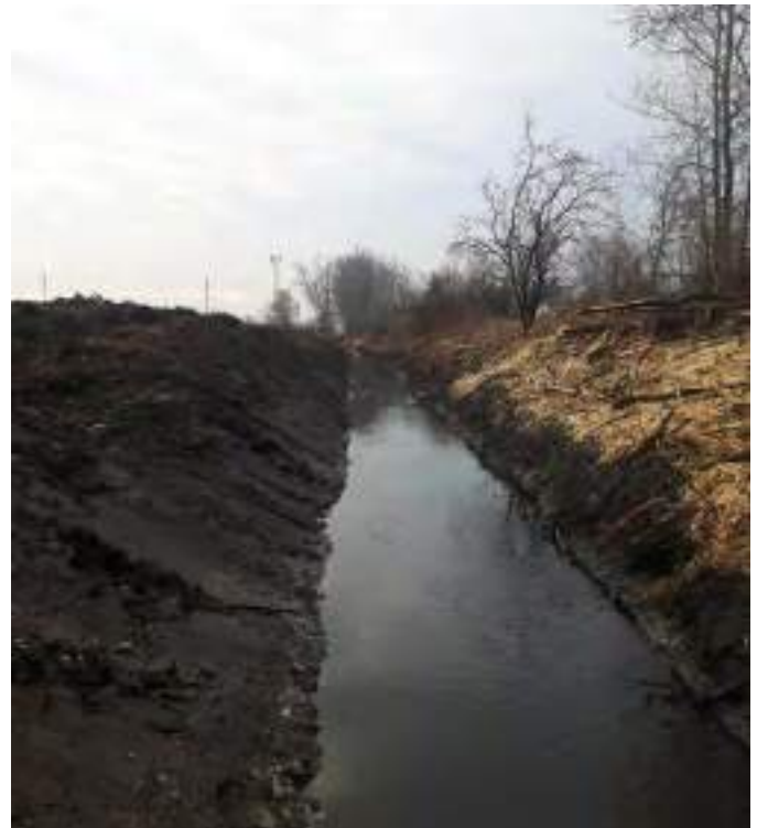
Figure A3-13. A recently completed full drain clean out. Source: Dietrich Engineering Ltd., Kitchener, Ontario
