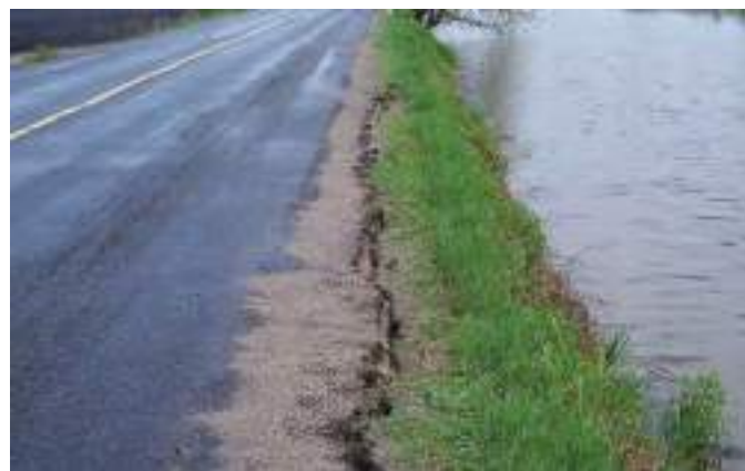
Figure A5-1. Investigation showing damage to a road along a drain.
