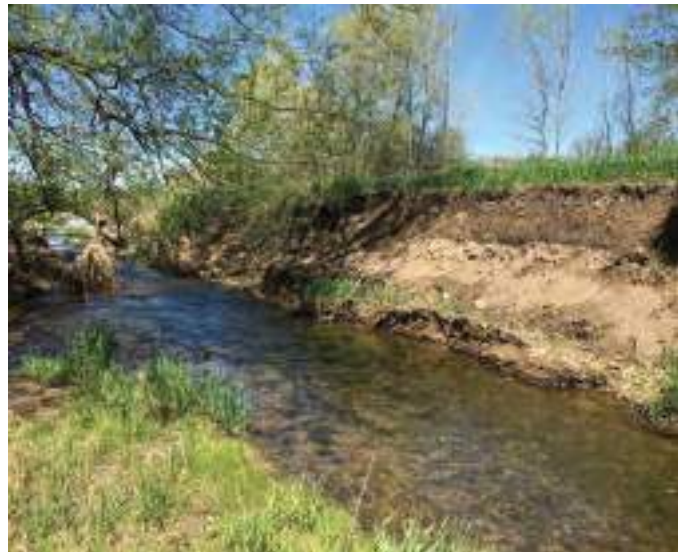
Figure B4-2. Bank failure along a drain.
