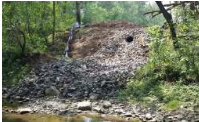
Figure A3-8. Bank stabilization and outlet repair. Source: Leroux Consultant, Municipality of Champlain, Ontario
