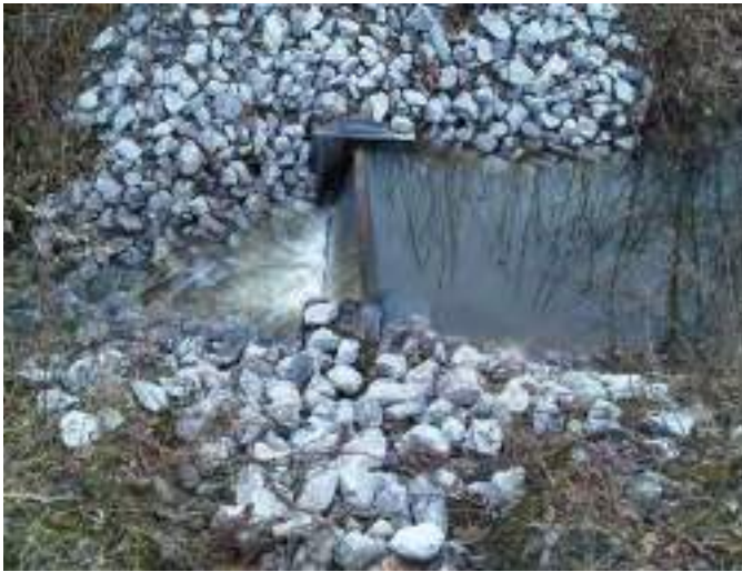
Figure B4-10. A water control structure (dam). Source: Dietrich Engineering Limited, Waterloo, Ontario
