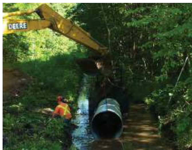
Figure B5-16. Dry Creek – installation of one of the water control structures.
