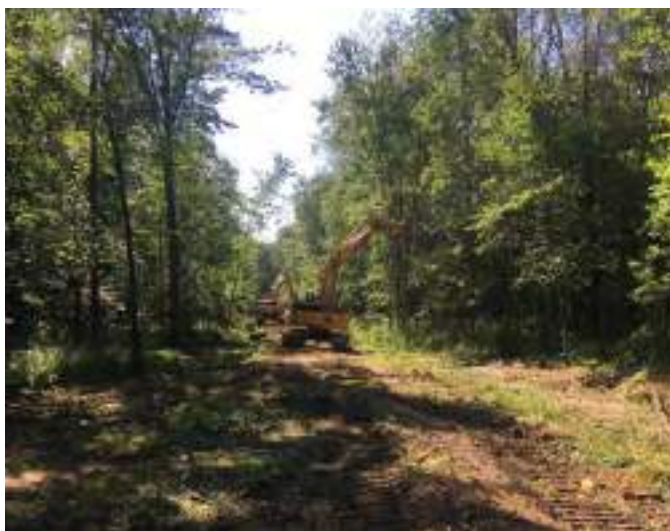
Figure A3-4. Brushing the top of a bank. Source: Dietrich Engineering Ltd., Kitchener, Ontario.
