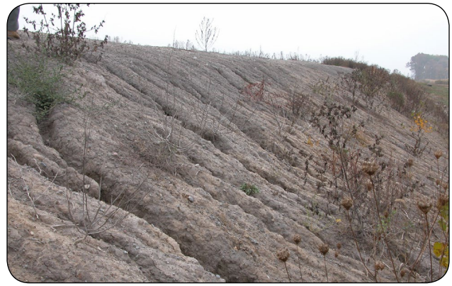
Figure 17. An example of a serious erosion problem because the bank was not re-seeded.
