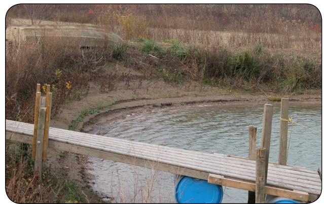
Figure 13. Wave action erosion at the high water level.
