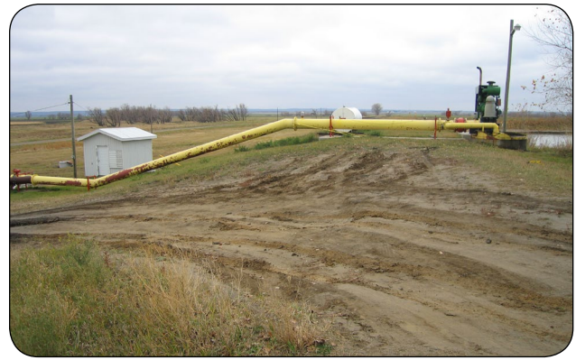
Figure 8. Pipes for filling and emptying the reservoir are placed over top of the berm (rather than through the berm).
