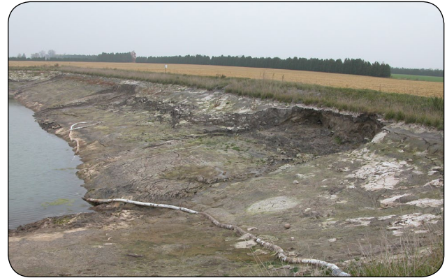
Figure 16. Failure and collapse of the interior bank of the reservoir.
