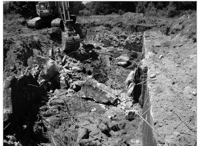
Figure 1. This unused manure tank is no longer environmentally sound. The excavator is in the process of demolishing and burying the structural materials on-site.
