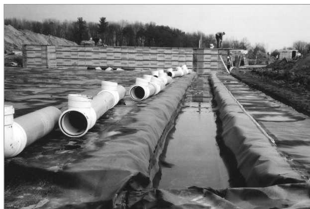
Figure 3. PVC pipe sections await connection and will eventually form a secure liquid manure transfer system from the in-barn tank to the external manure storage.
