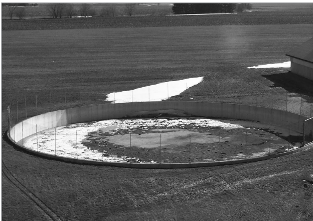
Figure 1. Open, circular, liquid tanks are commonly used on farms to store liquid nutrients such as manure from livestock operations.
