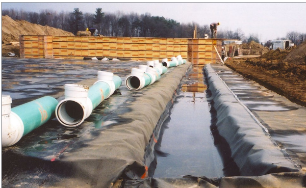
Figure 4. PVC pipe sections await connection and will eventually form a secure liquid manure transfer system from the in-barn tank to the external manure storage.
