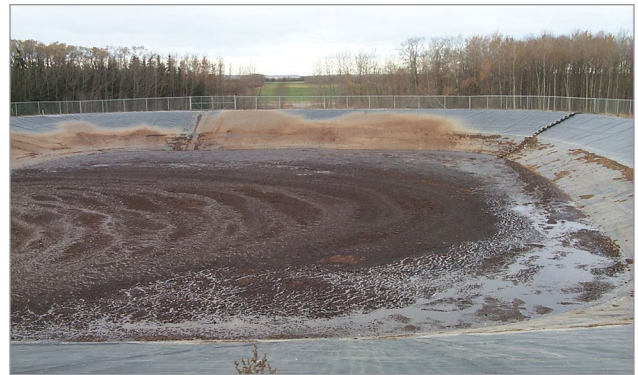
Figure 1. This earthen storage facility was constructed with a synthetic liner to provide the required protection for surface and ground water.
