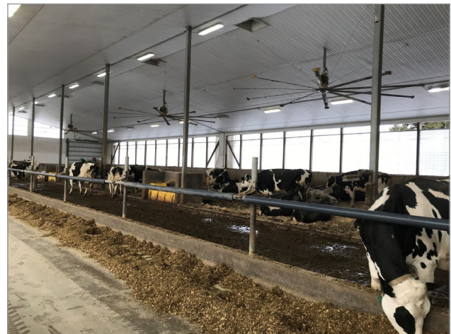
Figure 6. High-volume low-speed fans in a CBP barn.
