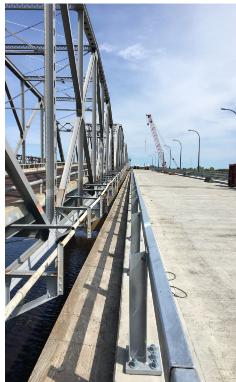
View of the narrow separation between the old bridge on the left and new bridge on the right.
