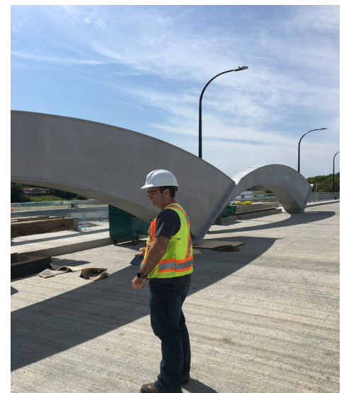
Tyler McQuaker (MTO) visually inspecting some of the arch segments prior to installation.
