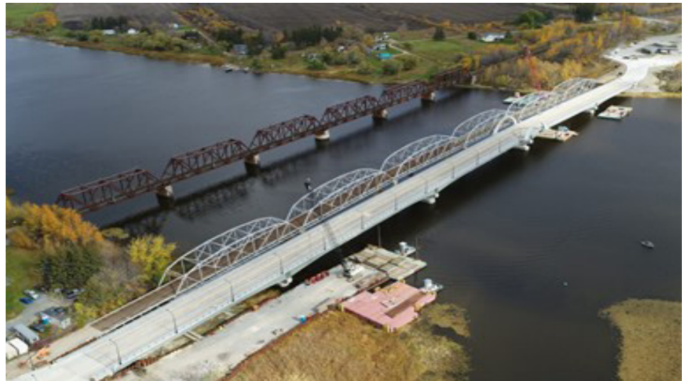
The new Baudette - Rainy River Bridge under construction, and the decommissioned 1958 Bridges, side by side.
