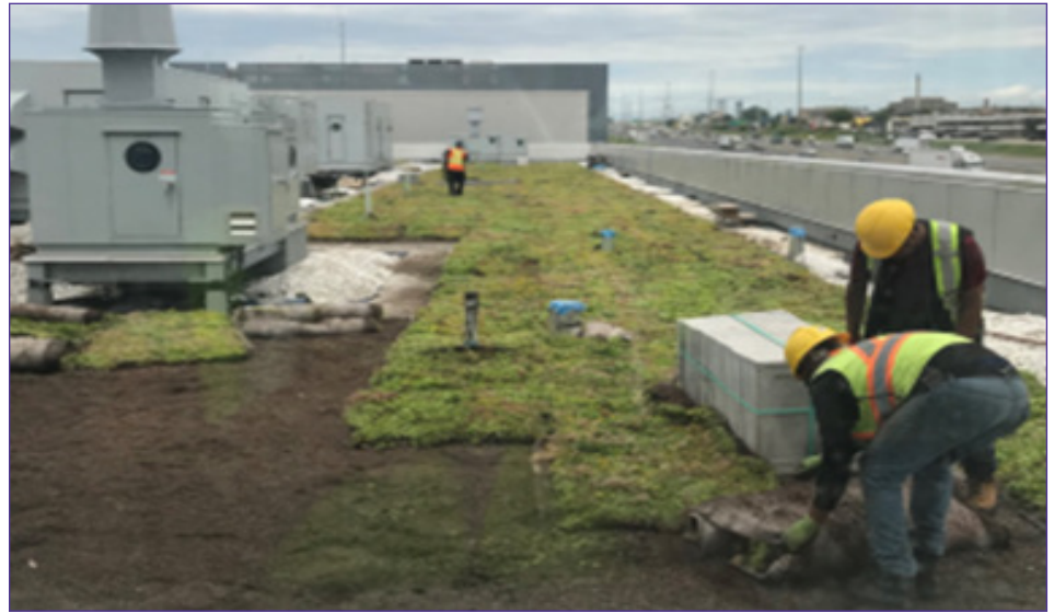
Installation of a green roof on the B-wing of the new CETI complex.
