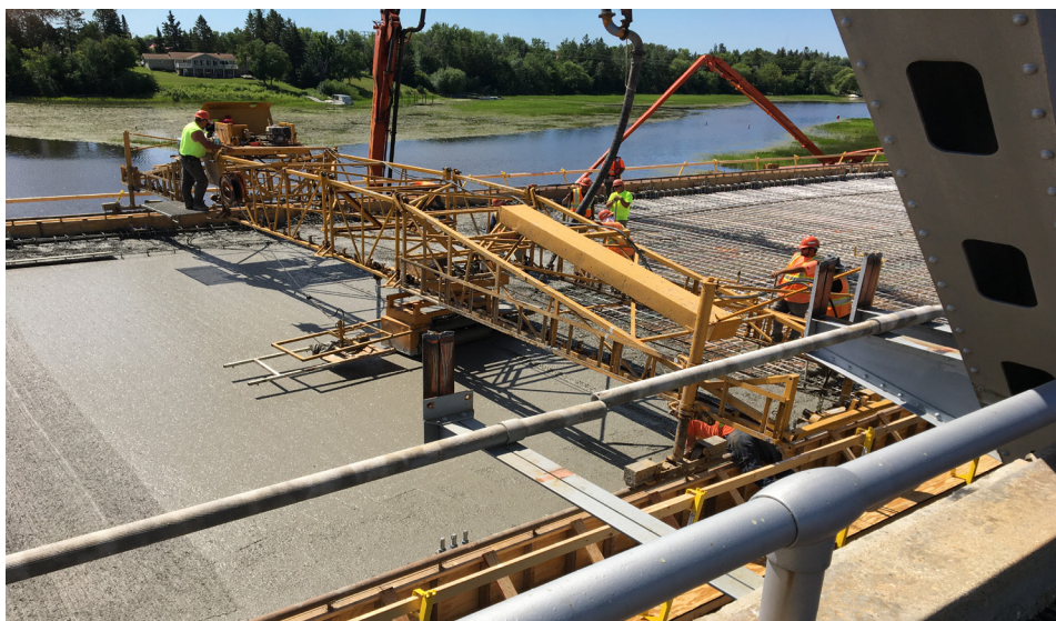
The contractor levelling concrete for the new cast-in-place bridge deck using a Bidwell screed machine.
