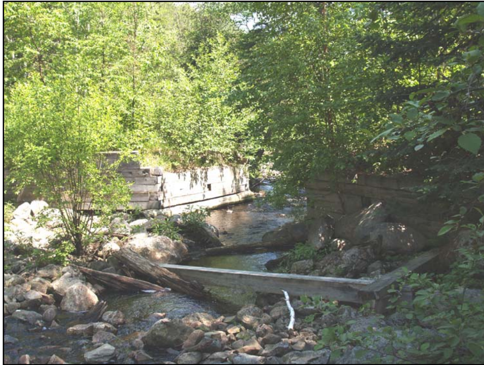
Photograph # 10. Bridge removed as an access control measure on the Owain Lake Road.
