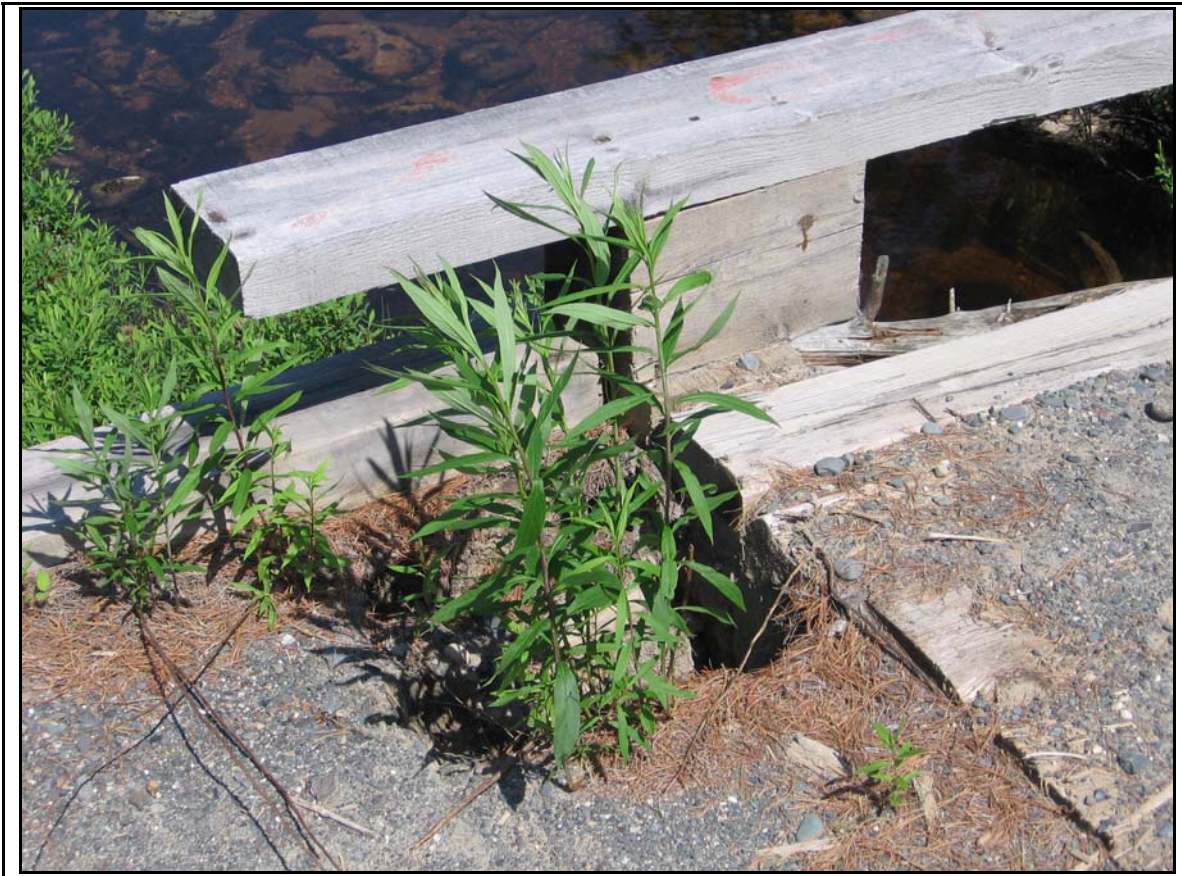
Photograph # 8. Weeds growing through hole in bridge – Blueberry Lake Block.
