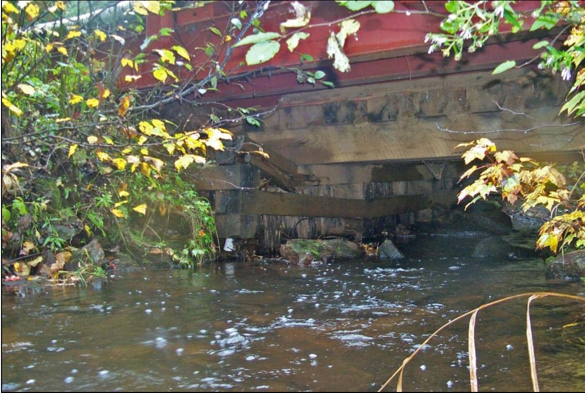
Figure 8. Temporary steel bridge over older wooden bridge allowed safe access and reduced stream sediments from old bridge until proper repair is made (Doorley Creek Rd.).
