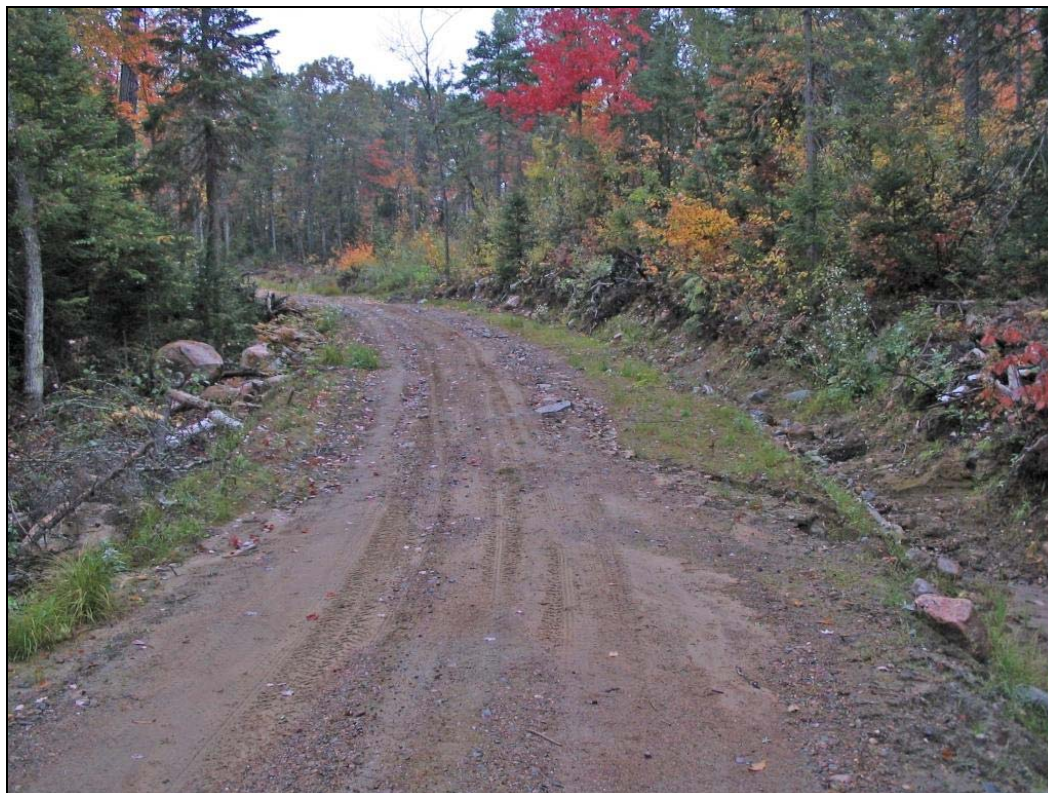
Figure 7. Erosion of the roadbed can be reduced by improved crowning, cross drainage, and ditching.
